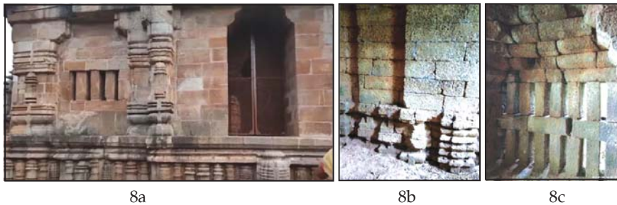
Figure 8 : (a) Base (vedibandha) moulding, stone jail and bevelled corbets in Lingaraj; (b) Base (vedibandha) moulding at Jinsar; (c) Stone jail and bevelled corbels at Jinsar
